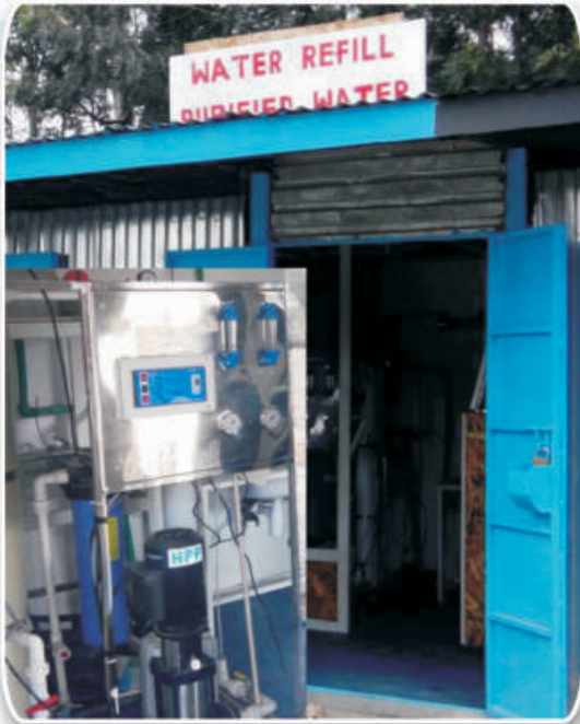
Photo shows affordable water kiosk in Kenyan rural area. It shows the front view of the kiosk and the filtration plant. (Installed By Indcare Africa)
